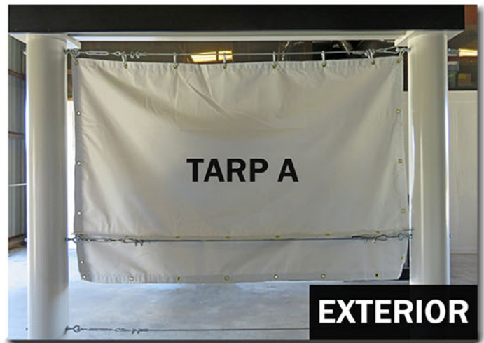
This is a view of Tarp A from outside the work area. It is also attached at its 1' opposite side overlap seam.
