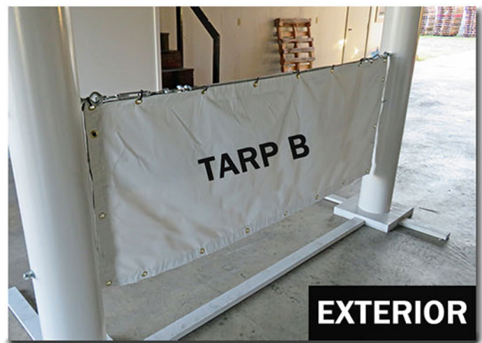
Tarp B is attached to the cable at the opposite side 1' overlap seam. This view is from outside the work area.
