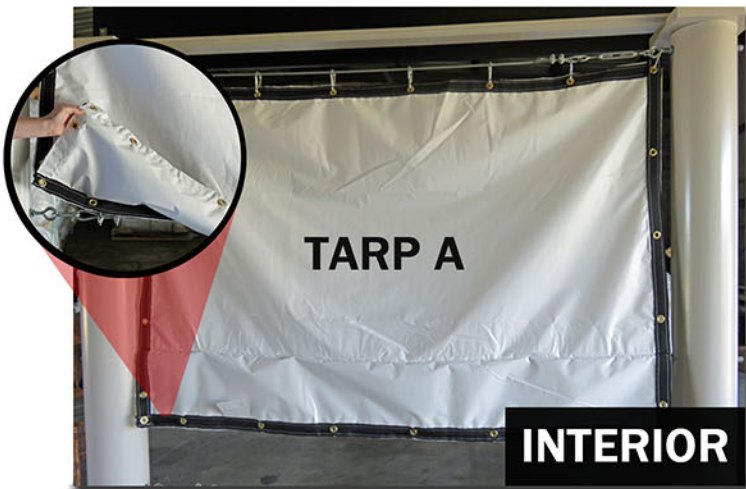
This is a view of Tarp A from inside the work area. It hangs from the cable at its top grommetted edge.
